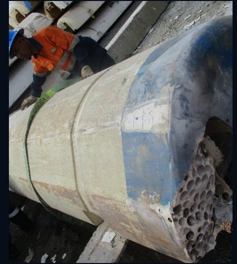
04 Damage found at inspection
